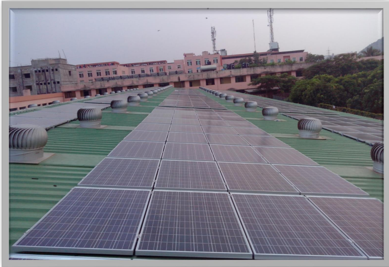
KALINGA INSTITUTE OF SOCIAL SCIENCES 500 KW SOLAR ROOFTOP INSTALLATION
